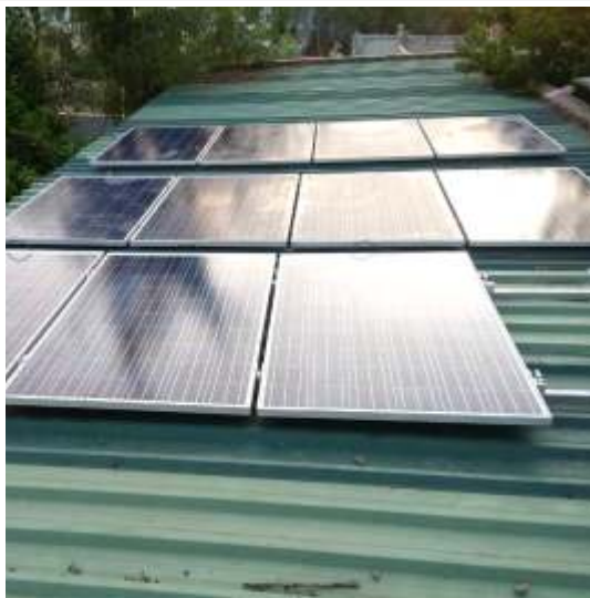
3 KW for Home at West Tambaram
